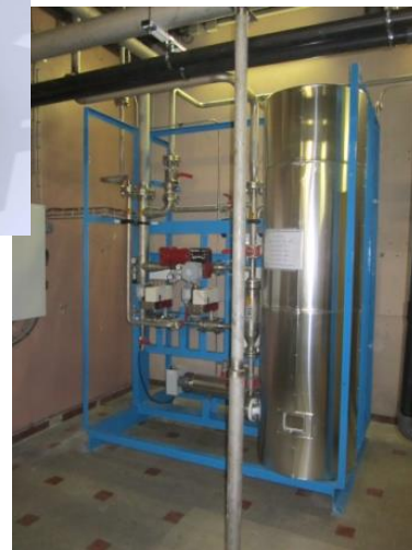
Oil removal system ( < 1 ppb C n H m )
