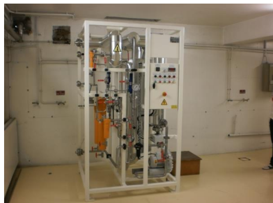
Continuous operation dryer ( < 1 ppm H 2 O )
