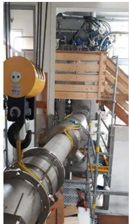
FIG. 3. View of the cryogenic line with in the background its connection to the cryogenic satellite.
