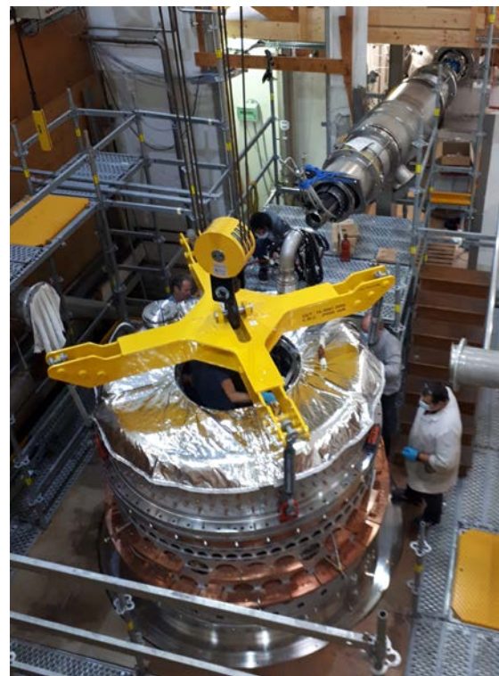
FIG. 3. Installation of the cold mass with its first layers of superinsulation on the support ferrule of the cryostat.
