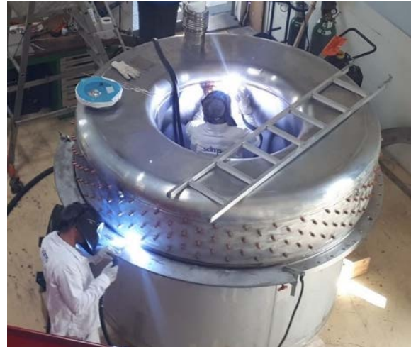
FIG. 2. Closure welding of the He vessel with the superconducting coil inside requiring a strict control of the temperature to not damage the electrical insulation (contractor SDMS).
