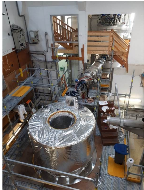
FIG. 2. Last superinsulation layers covering the 100 K thermal shield installed prior to the mounting of the outer vacuum chamber.
