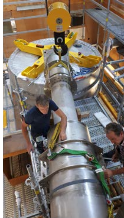
FIG. 2. Fixation of cryogenic line to its support foot. In the background, the connection to the magnet cryostat.
