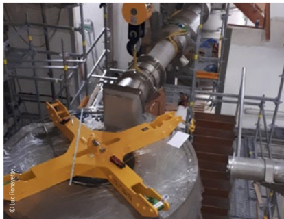
› Figure 3: Trial assembly of the cryogenic line (contractor Cryo Diffusion) connecting the cryogenic satellite in the back to the superconducting magnet cryostat in the front.
